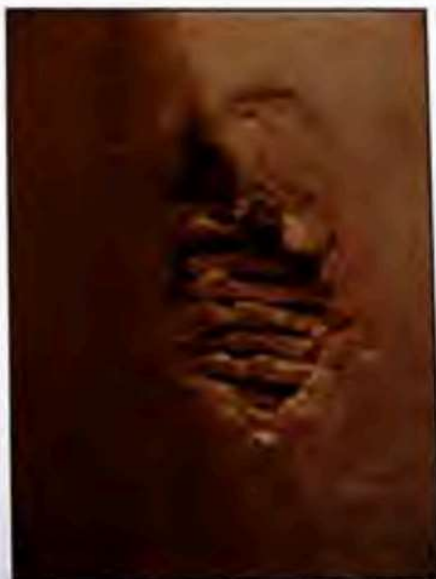
Sample of hole dug into the wall with lath showing
